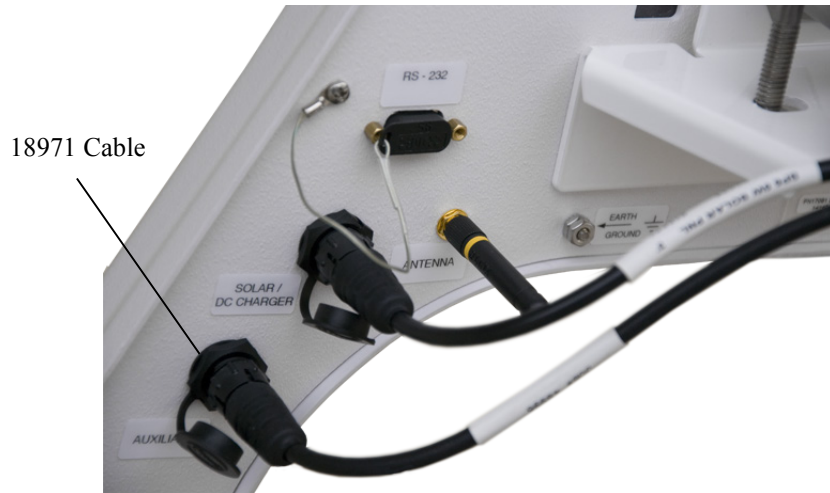
FIGURE 5-23. 18971 cable connected to WS-PRO LT station
